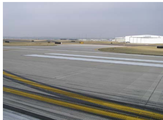
(Figure 20) Taxiway Lead in lines Centerline Extending to the Runway Centerline
