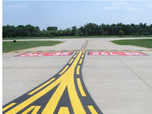
Figure 8b : Enhanced Taxiway Centerline
